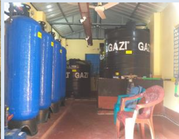
Water treatment facilities in the plant
