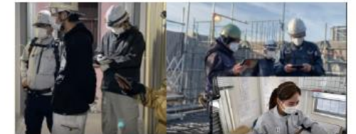
Attendants can participate in online morning assemblies using a smartphone. (Left: interior contractor; top right: frame contractor; bottom right: on-site office)
