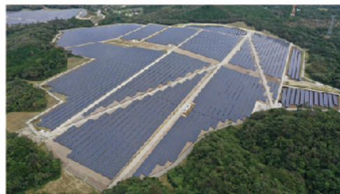
“Matsushima-Donguri Solar Power Plant,” boasting 50 MW panel output
